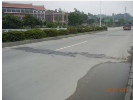
Fig. 16 The damaged pavement around the top of link slab
