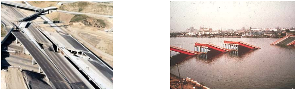
Figure 1. Unseating of non-integral spans in the San Fernando 1971 (left) and Niigata 1964 (right) earthquakes.
