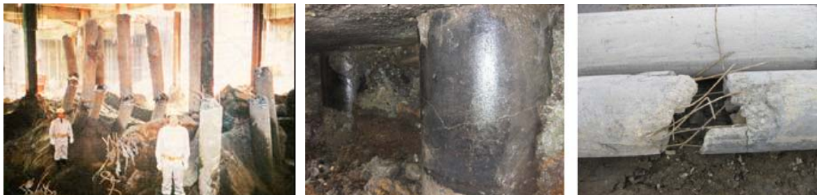
Figure 13. Piles failures during earthquakes (Tohoku earthquake).
